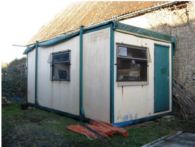
The Portacabin, with a tarpaulin protecting its roof
